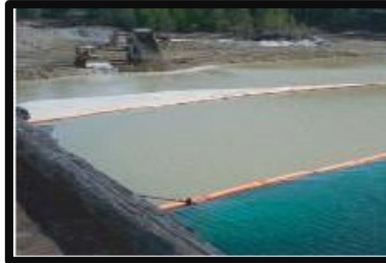
Double impermeable curtain system with oil absorbent boom in use in a lake at a mine reclamation site.
